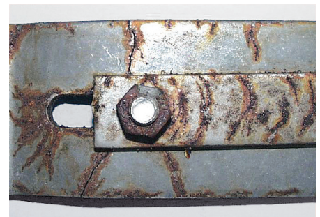
Fig. 8: SCC of a bracket made of the material 1.4301 (A2, 304) after approx. 4 years of use in an indoor swimming pool.
